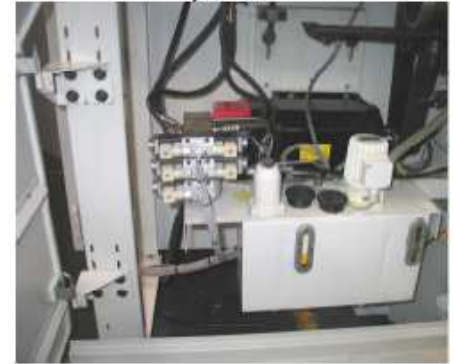
Completely new hydraulic system
